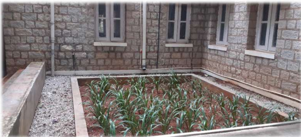
Rainwater Harvesting unit
