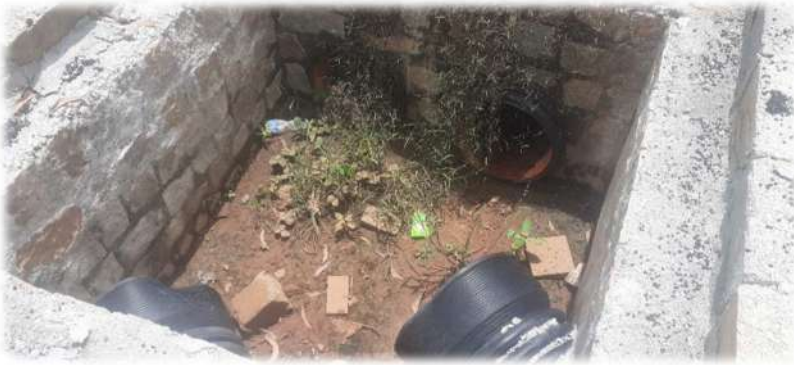
Conducts to carry Rainwater from rooftop to rainwater harvesting pond
