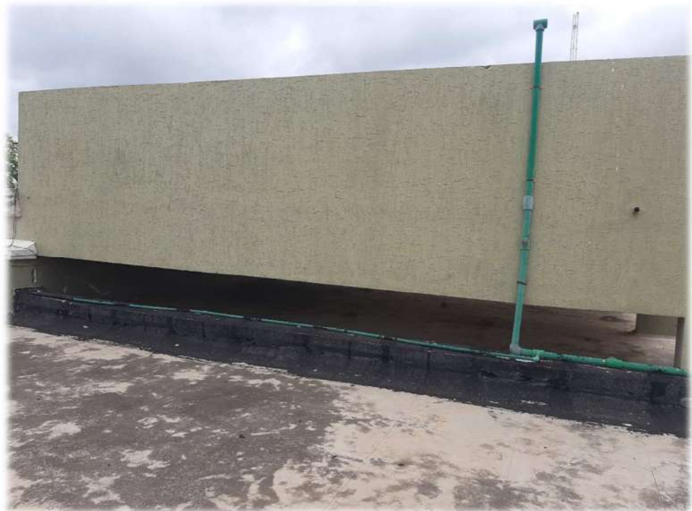
Overhead water storage tank
