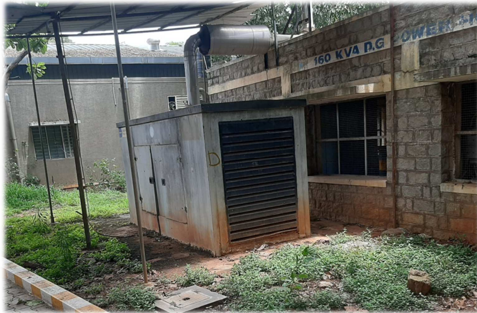
Diesel Generator (alternate source) during power cut
